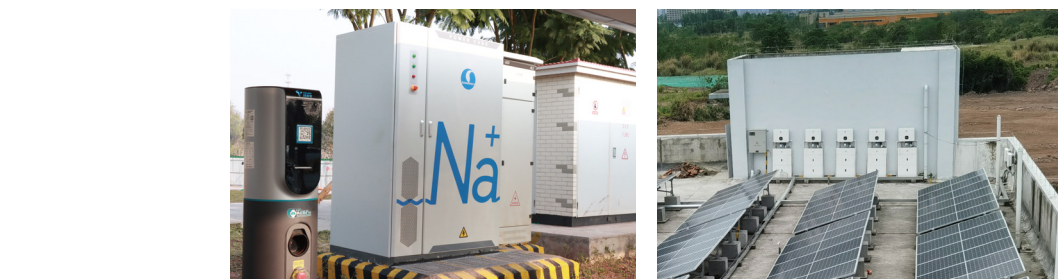
NaESS+PV+Charger Integration Project
