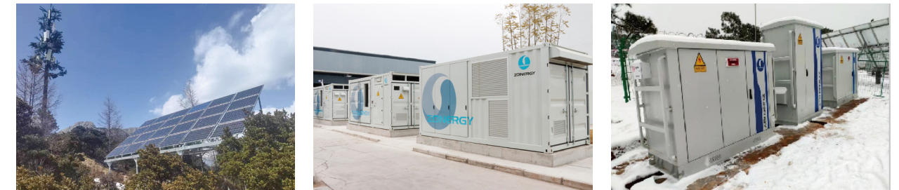
Telecom base applicaiton
