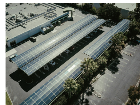
Photovoltaic Energy Storage and Charging Station
