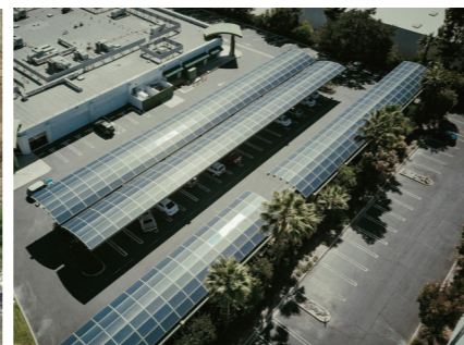
Photovoltaic Energy Storage and Charging Station
