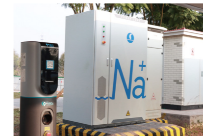
NaESS+PV+Charger Integration Project
